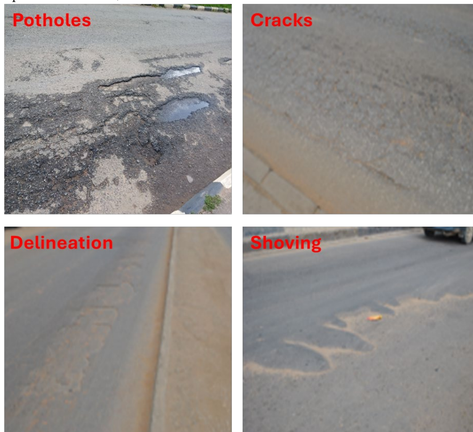
Plate 1: Pavement distress observed on the road
