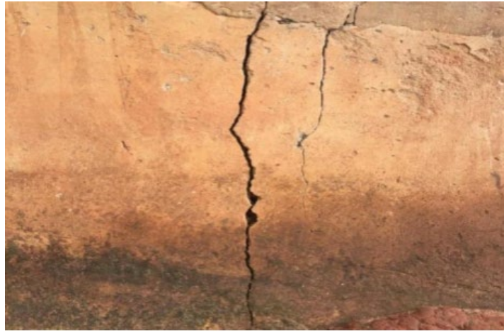
Figure 5: Cracked Wall in Magashanu Community due to Granite Quarrying
