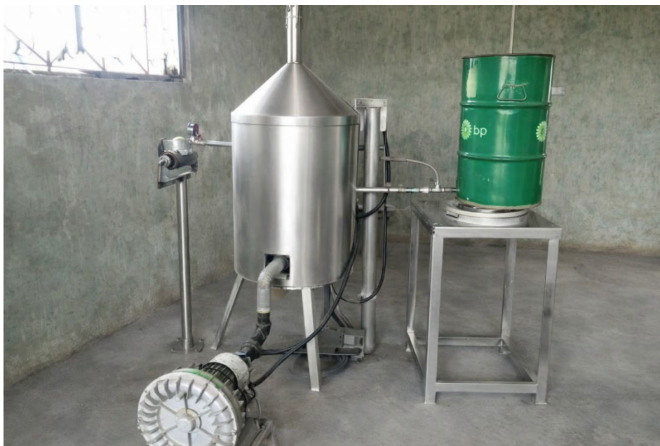
Figure 2: The fabricated steam generation system
